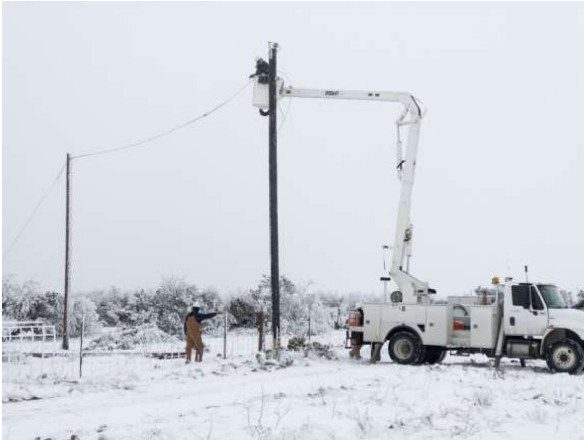
Linemen work to restore power in Pecan Mott, Texas. Photo: Jonathan Cutrer
